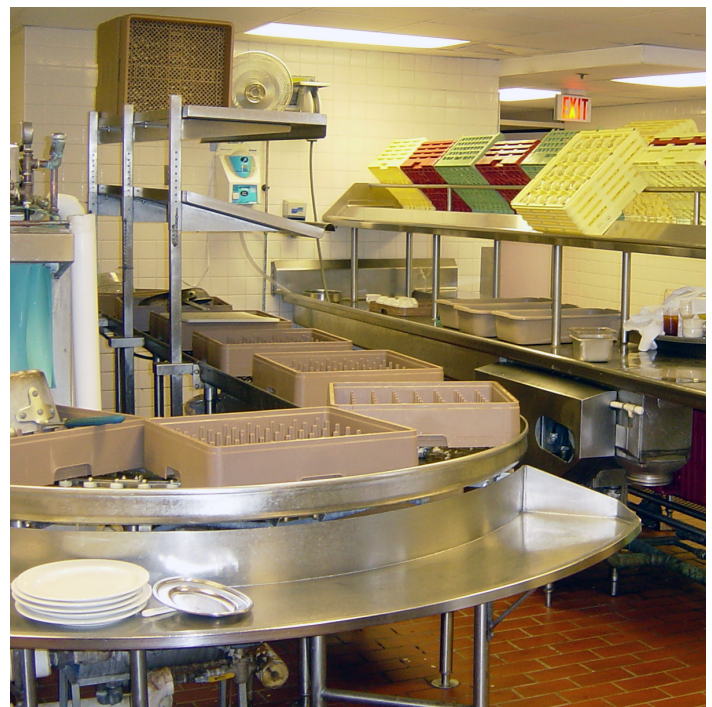
▼ Insinger Rack-A-Matic dishwashing system at The Statler Hotel.
