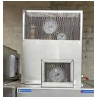
Stainless steel perforated boxes are used to protect the thermometers and gauges from damage.
